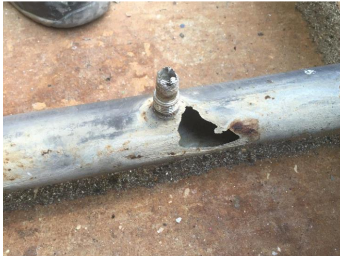
Figure 9: Wear damage of carbon steel tube.
