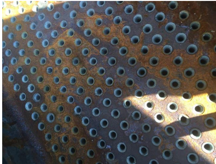
Figure 7: Corrosion of the stainless steel tube sheet.
