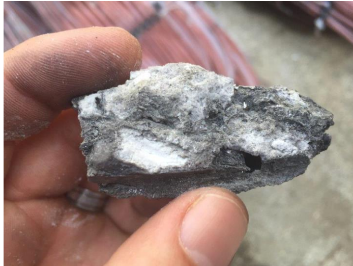
Figure 8: Fly Ash build-up retrieved from the tubes during maintenance.
